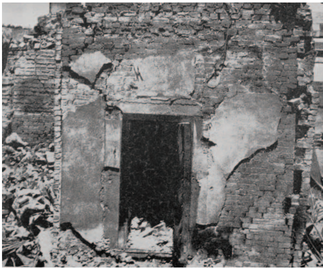
Bank of New Zealand stong room that was no so fortunate. Image source: Geoff Conly, Hawke's Bay Before and After: The Great Earthquake of 1931: An Historical Record , Daily Telegraph, Napier, 1981, at page 124.
