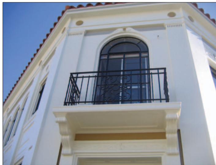
Italianette balcony over the front entrance to the building. Image source: Sainsbury Logan & Williams Archive.
