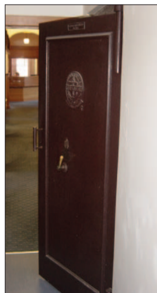
View of strong room door looking down the hallway towards reception and the exterior door. Image source: Howard Bott (Practice Manager).
